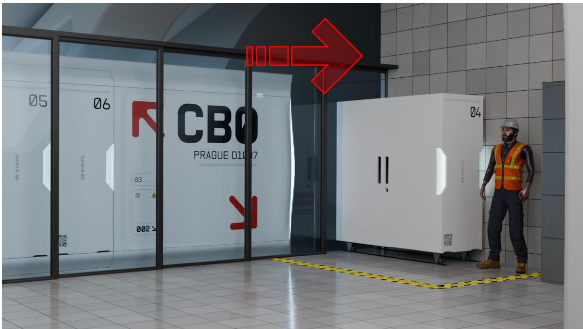
Fig. 6-19 Platform screen door closing after unloading
